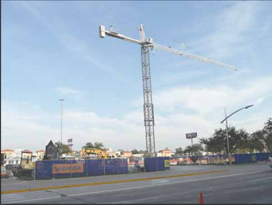
Capp Electric Co. is the electrical contractor at a Class A office building project on Post Oak Blvd. The GC is Skanska USA . -ab
