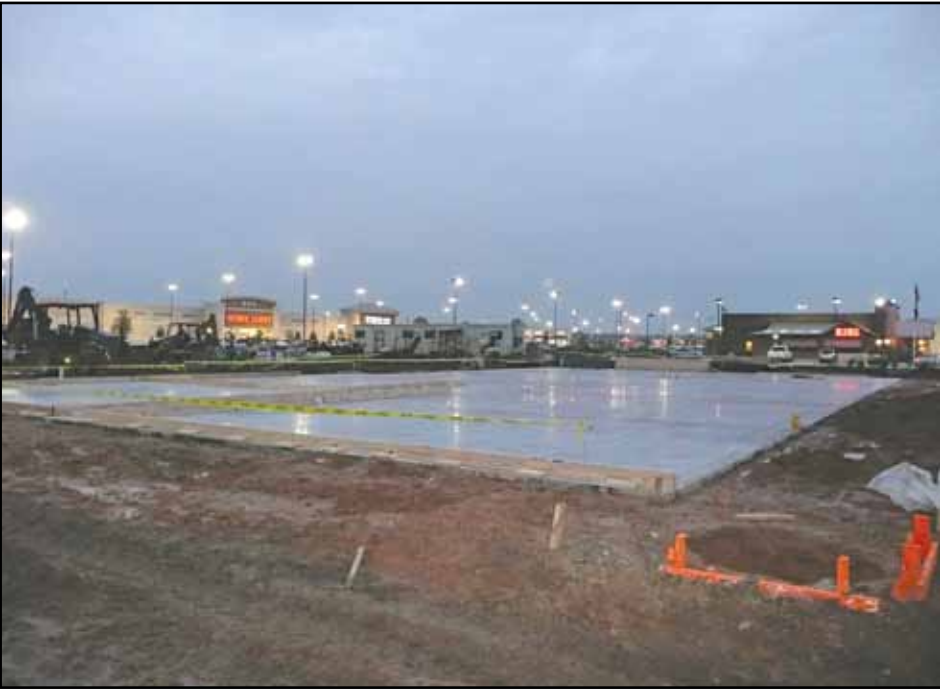
Gamma Construction is the GC at the 2630 Gulf Freeway project in League City, TX. -ab
