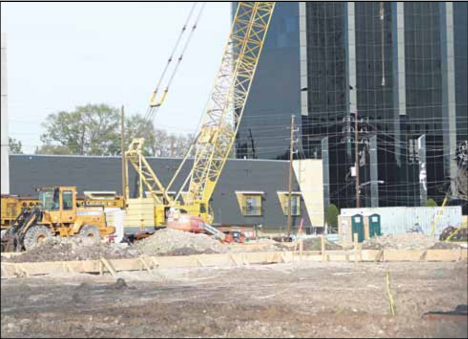
STILLC is the concrete contractor at the 3788 Richmond project near the Galleria area. Morgan Group is the GC. -ab
