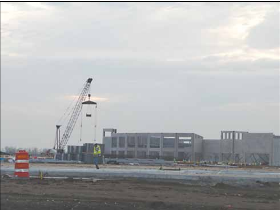
Hardin Construction is the GC at the Tanger Factory Outlet Center project in Texas City, TX. -ab
